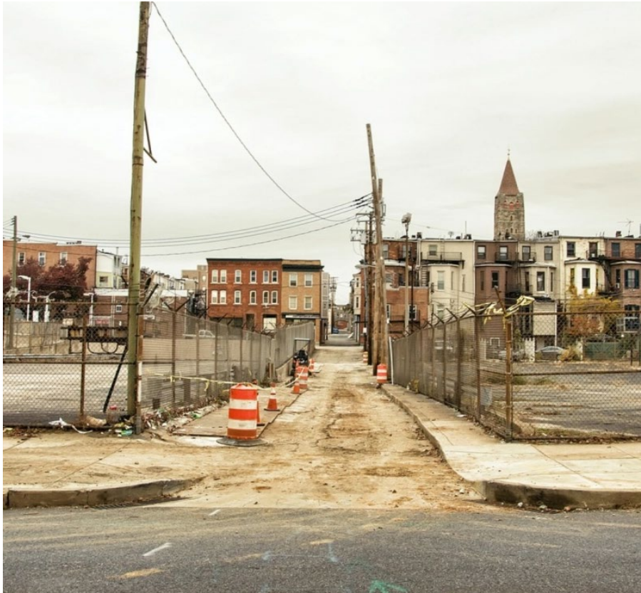
A street in North Baltimore, Md. with a badly damaged sidewalk. A series of orange construction barrels mark an uneven segment of alleyway pavement between two curb cuts that is filled with dried mud and would likely be impassible to many people using assistive devices. Parking lots and brick row homes stand in the background.
