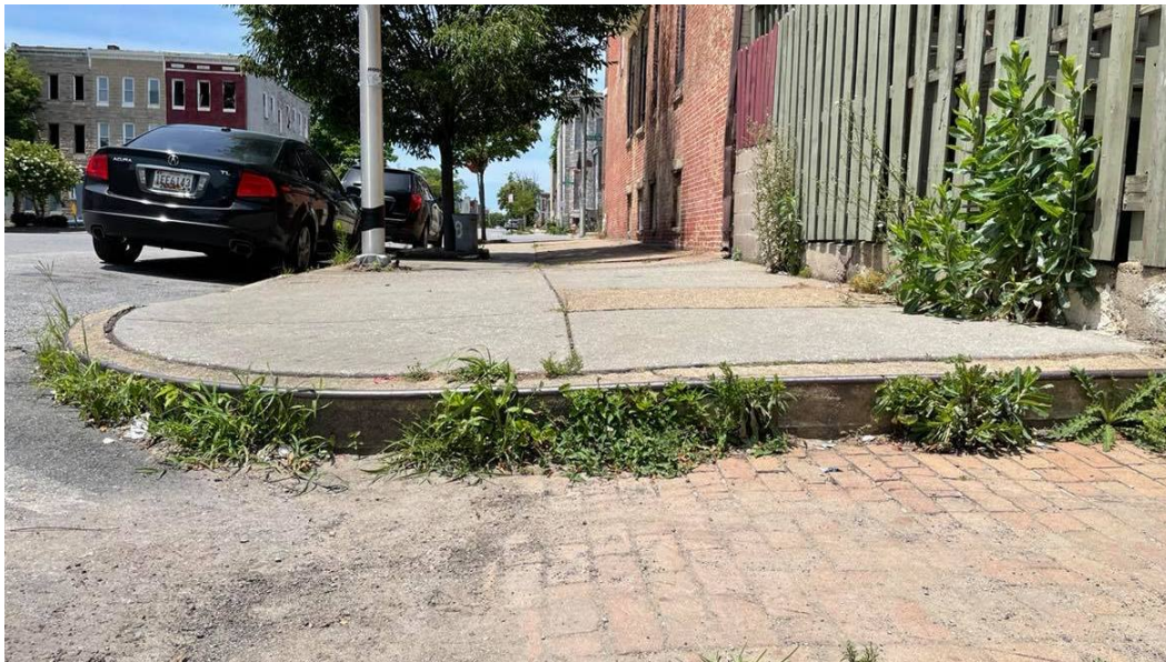
No curb ramp at all at this spot on Westwood Avenue in West Baltimore. (Fern Shen)
